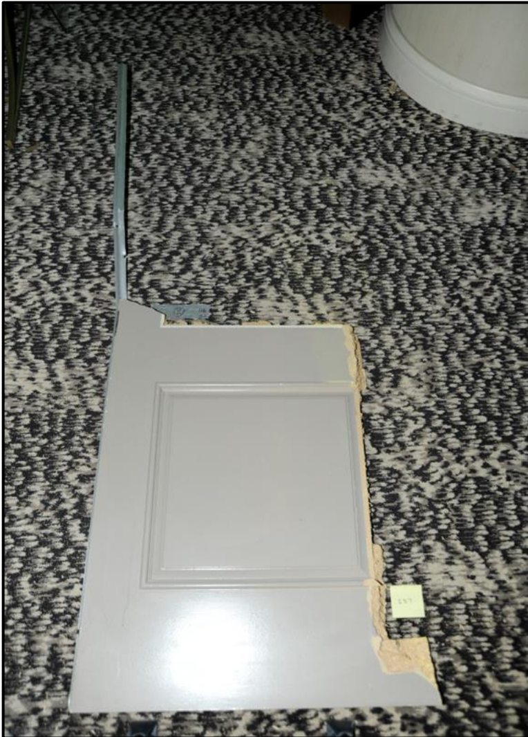
(Damage to entry door of room 32-135)
