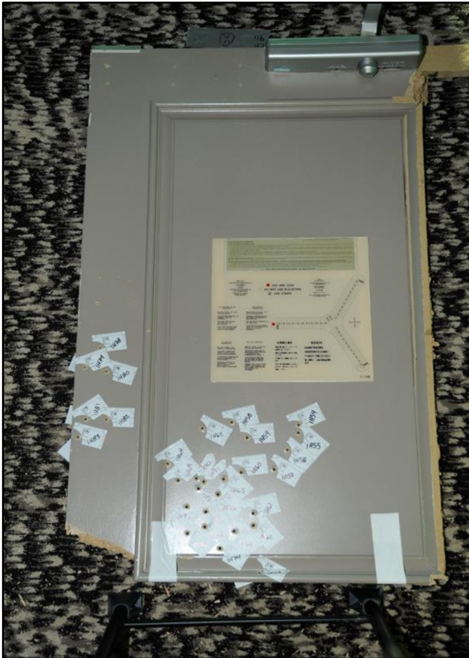
(Damage to entry door of room 32-135)
